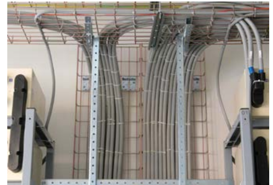
▲ Cloth cable installed in a Central Office.
